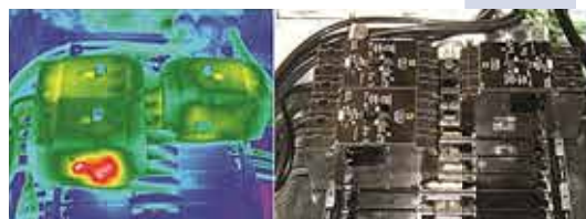
IR problem sample ( Internat contact of a circuit breake )
