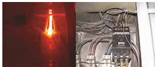
IR problem sample ( wire termination )
